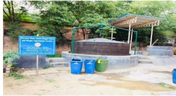
View of anaerobic digester running on kitchen waste
